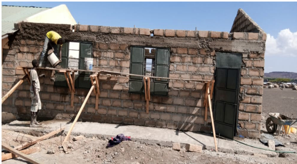
Shalom-SCRR funded Classrooms block at Santur Primary School, in Marsabit, Northern Kenya, set up to provide learning spaces to more than 370 girls and boys who live under extreme poverty and marginalization that impedes their potential in academic success.
