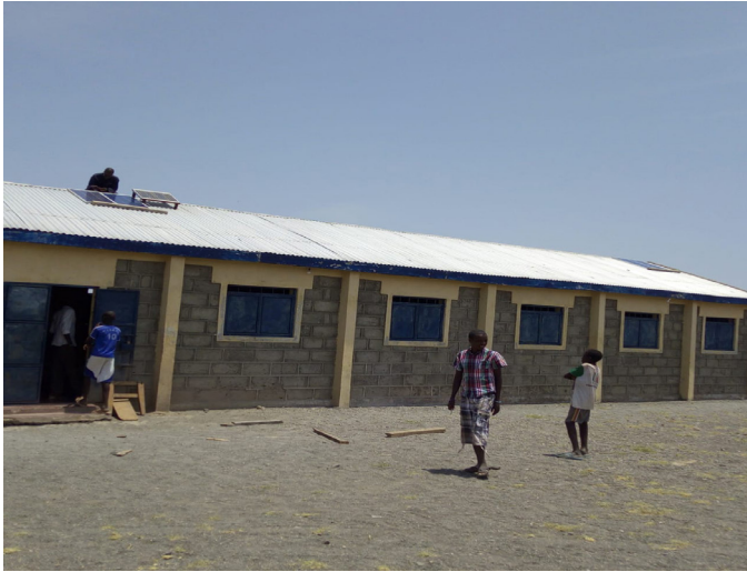
Solar System installation in one of the marginalized schools in Northern Kenya funded by Shalom-SCCRR to provide lighting for both the pupils and the school administration.
