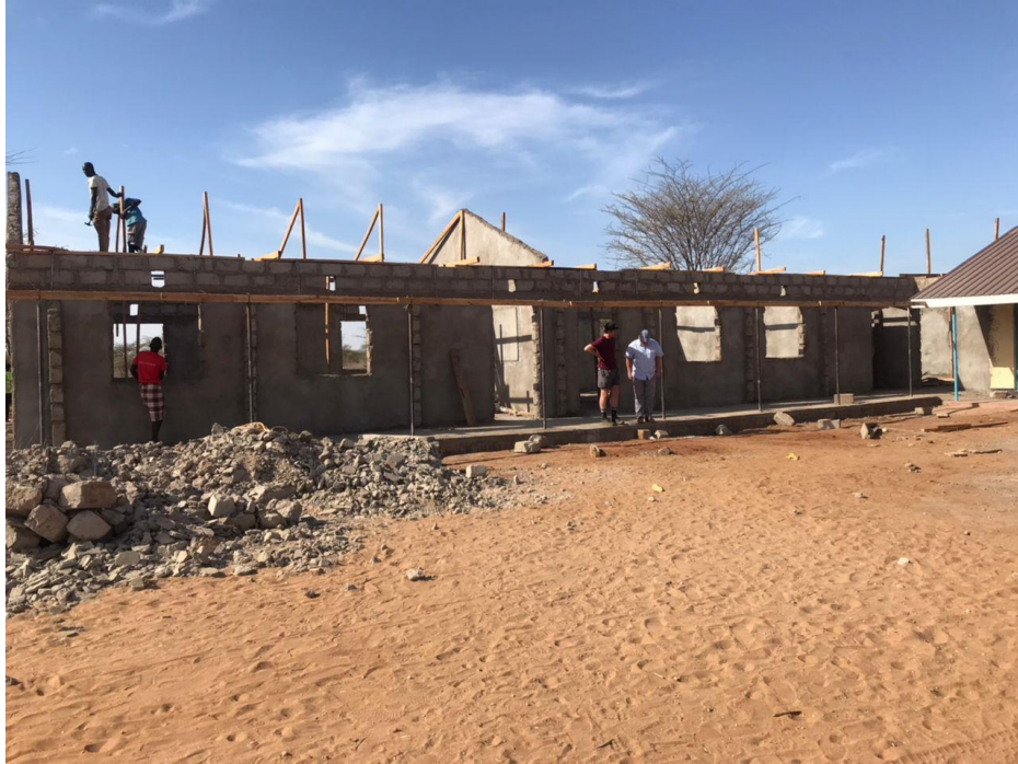
Fr. Oliver Noonan MA, shalom-SCCRR Executive Director with Mr. Ciaran King assessing the progress of Shalom-SCCRR funded classrooms construction project at St. Peter's Nursery and Primary School, Turkana County
