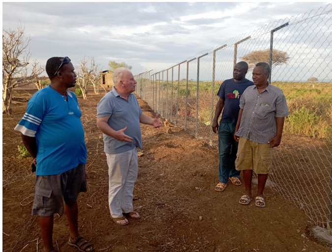
Fr. Oliver Noonan MA (PhD Candidate) and Mr. Arthur Magero MA, project officer, assessing a fence installation and other construction projects for schools/educational development in a remote area at the Kenya-Ethiopia volatile border .
