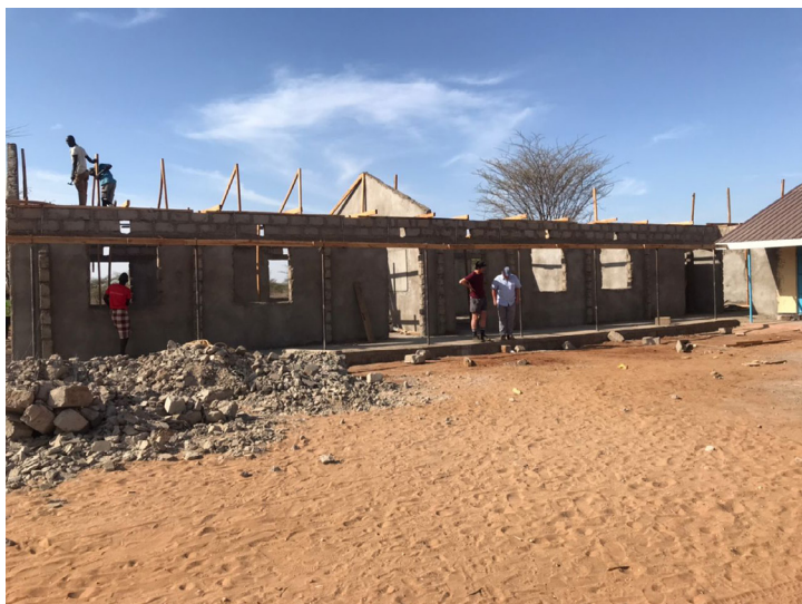
Shalom-SCCRR's Executive Director, Fr. Oliver Noonan MA (PhD. Candidate) and Mr. Ciaran King, witnessing an ongoing construction of classrooms funded by Shalom-SCCRR in Turkana County, Kenya.
