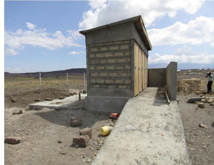
Construction of standard latrines/toilets: Good latrine conditions at school have improved the school environment by meeting specific health and hygiene/sanitation needs of both boys and girls and to a significant extent reducing absenteeism .
